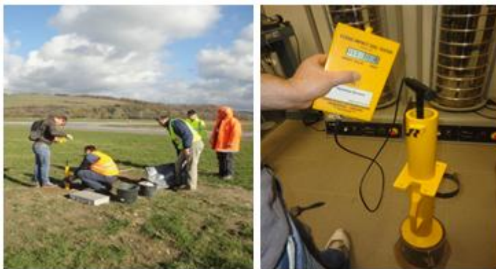
Figure 9. Control of compaction rate by Clegg Impact Soil Tester for on clayey gravel
