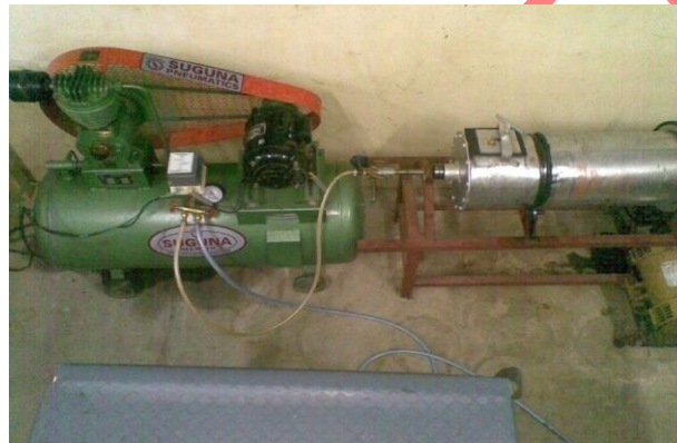
Fig. 2. Rotary Stainless Steel drum covered with an insulation of 25mm rigid polyurethane cast in-situ material well tucked in-between steel pipe and anodized sheet
